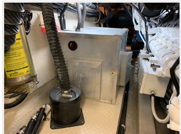
2nd Gen Set Engine Room
