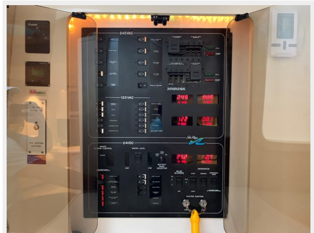
Breaker Panel at Entry to Below
