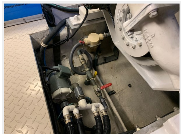
Engine Room Bilges
