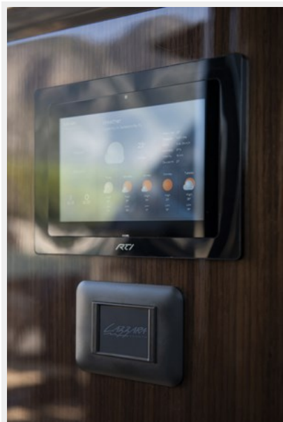
RTI lights and curtains automation
