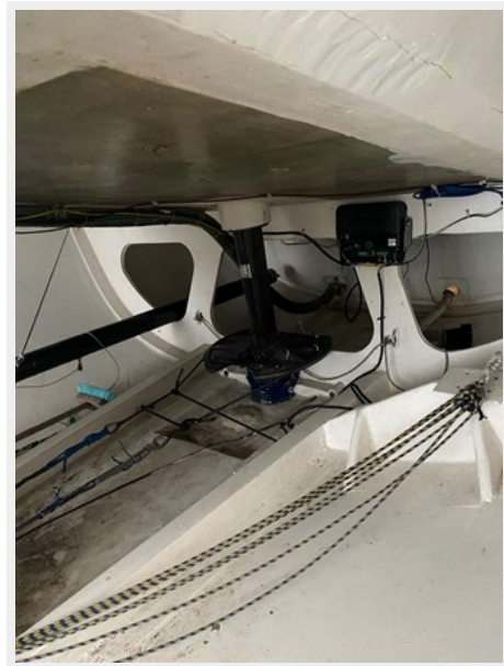
Under cockpit - systems IMG_3592
