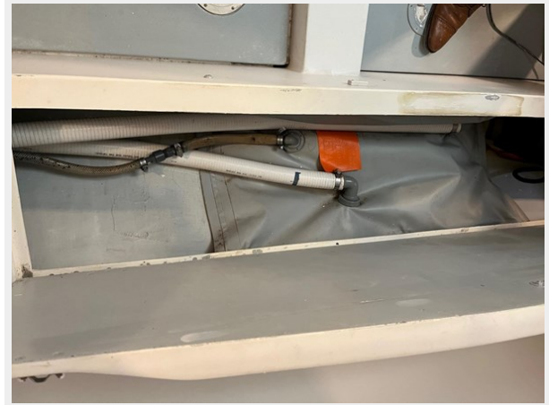
Water bladder tank IMG_1843
