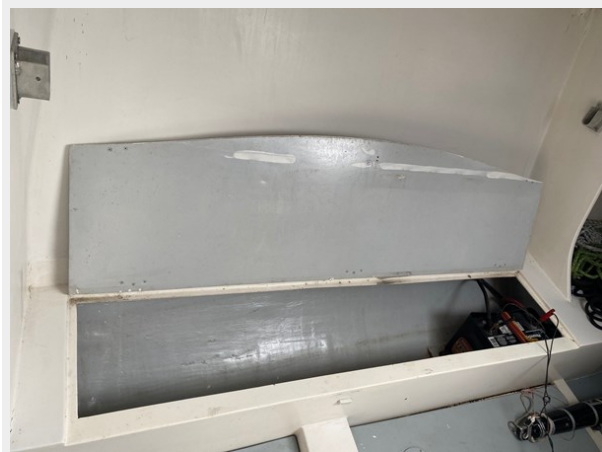
Battery - under bunk stbd IMG_3577
