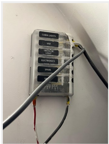
Junction box V-berth bulkhead IMG_1851
