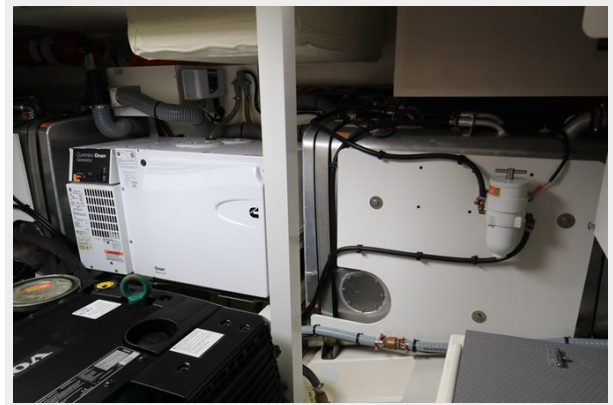
20 Engine Room Generator
