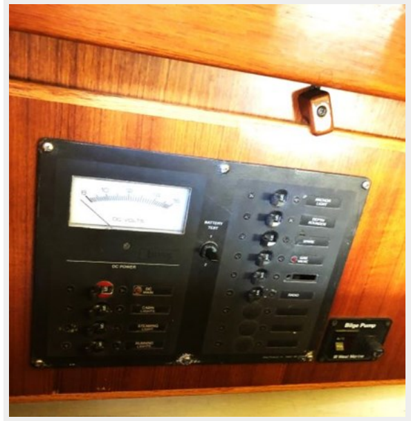
DC electrical panel IMG_9610
