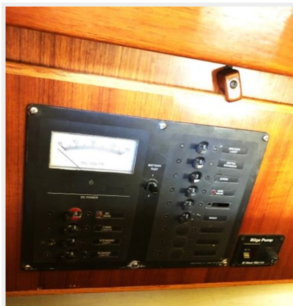
DC electrical panel IMG_9610
