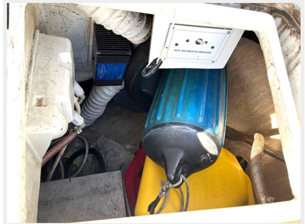
Lazarette - breaker & shower IMG_1746
