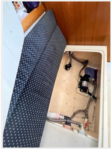
Freshwater pump IMG_1758
