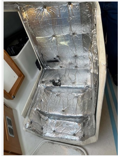
Engine insulation IMG_1782
