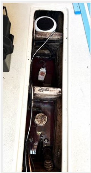
Fluxgate compass in bilge IMG_1780
