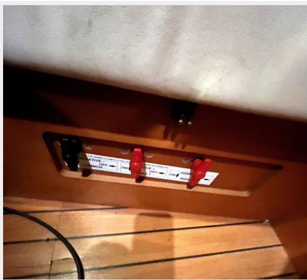
Port settee & battery selectors IMG_2101
