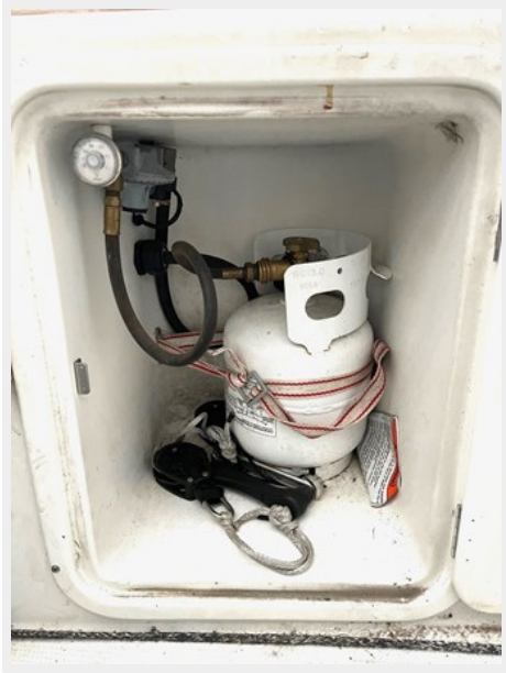
Propane locker & tank IMG_2091
