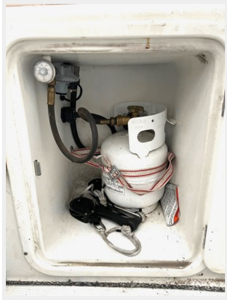
Propane locker & tank IMG_2091
