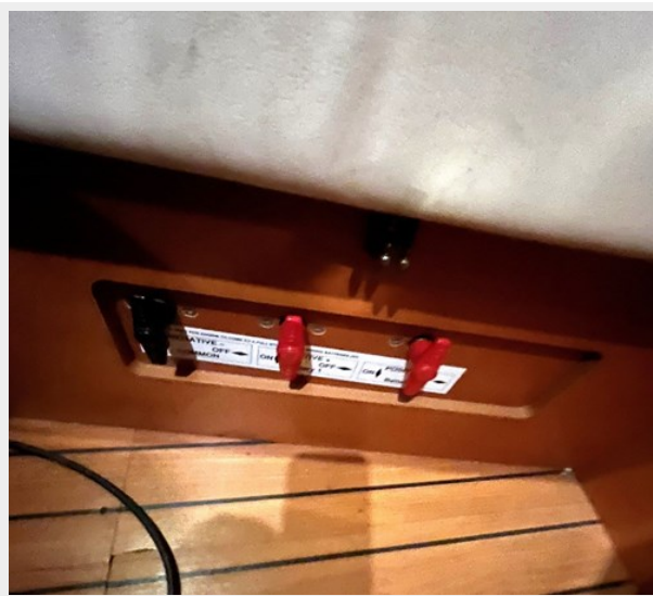
Port settee & battery selectors IMG_2101
