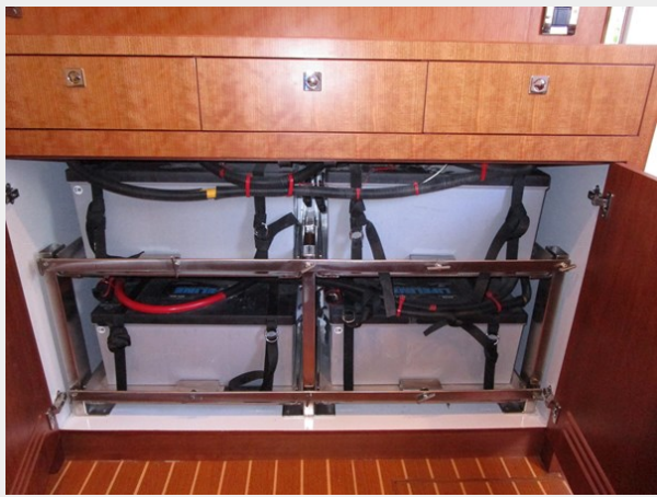
House battery sliding access
