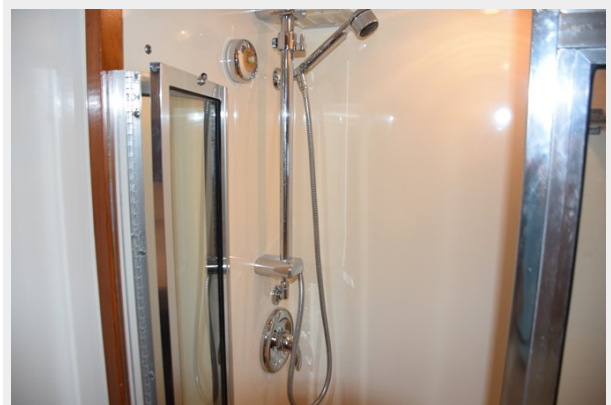
Shower, New Mixer Fixture
