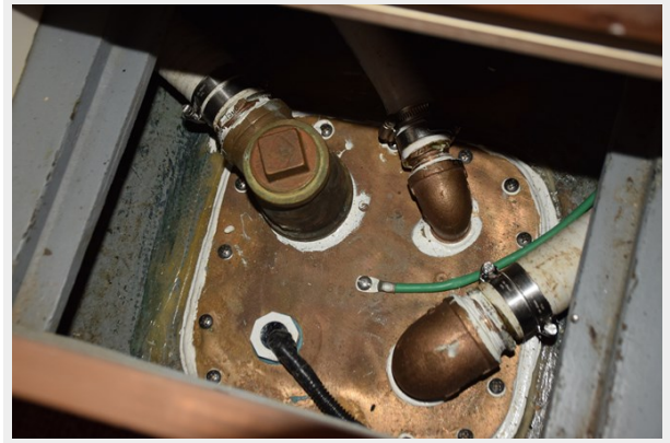
All New Holding Tank Plumbing
