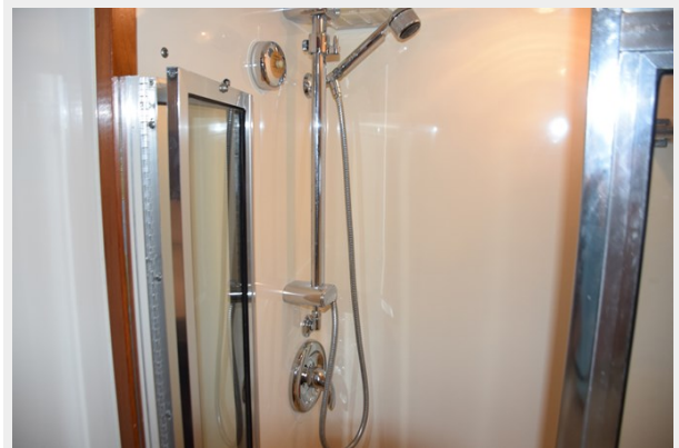
Shower, New Mixer Fixture
