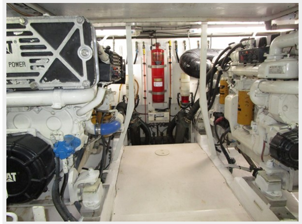
Engine Room Looking Fwd.
