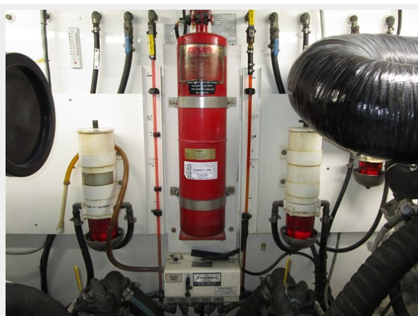
Engine Room Forward
