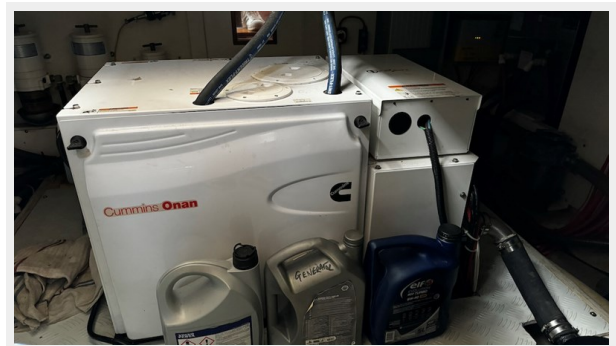
Engine room generator
