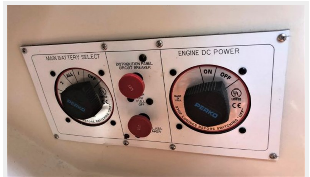
Battery selector switches & breakers IMG_5161
