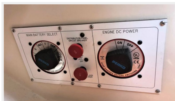
Battery selector switches & breakers IMG_5161
