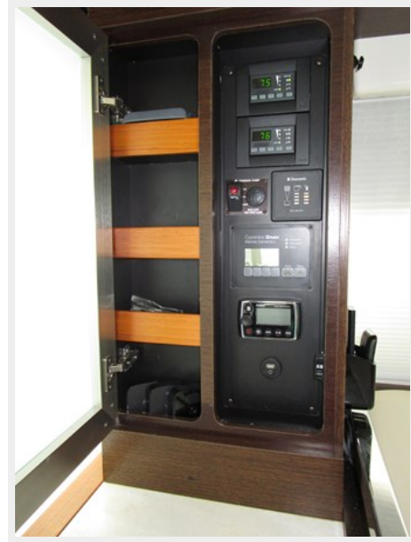
Upper Control Panel
