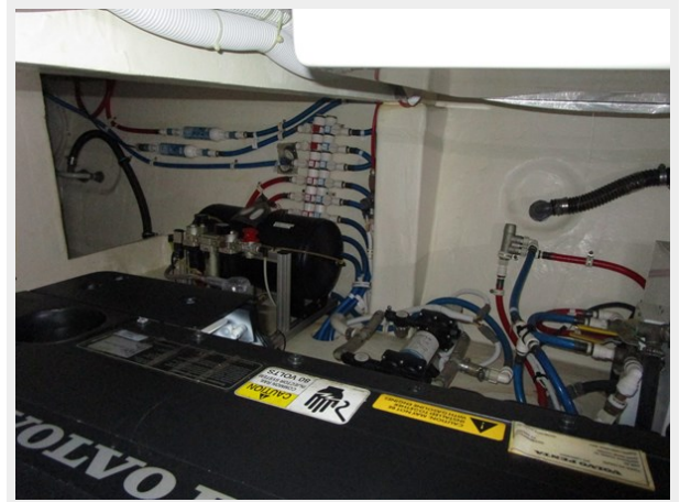
Port Side of Engine Room
