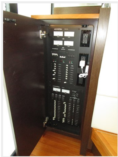
Lower Electrical Panel
