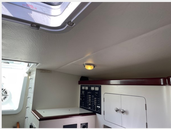
Cabin Aft-Electrical Panel & Storage
