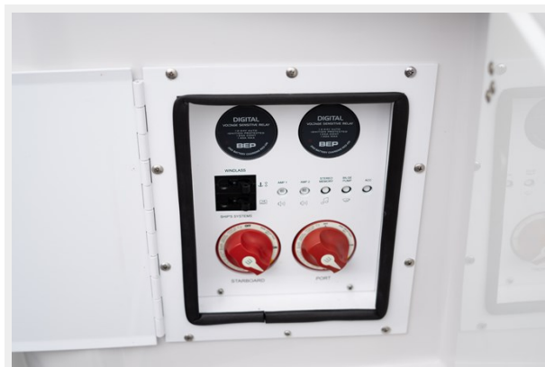
26. h290 battery switches
