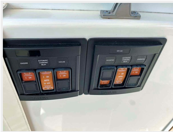
Remote Battery Switches at Helm
