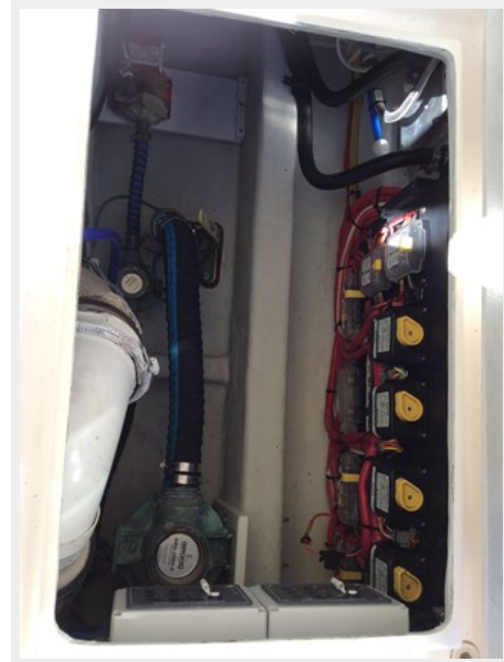
Engine Room, Day Hatch Access
