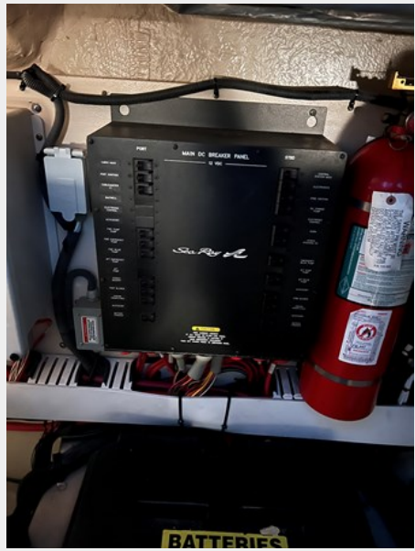
Main DC breaker panel
