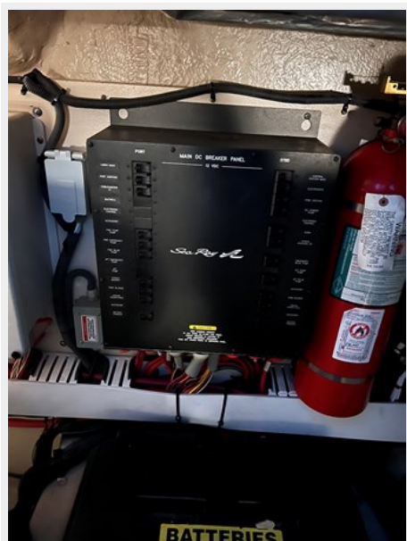
Main DC breaker panel
