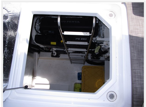
Engine Room Entrance
