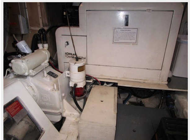
Engine Room Forward
