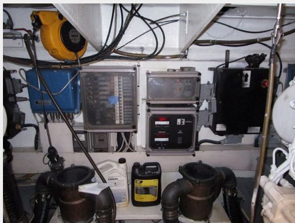
Engine Room Aft
