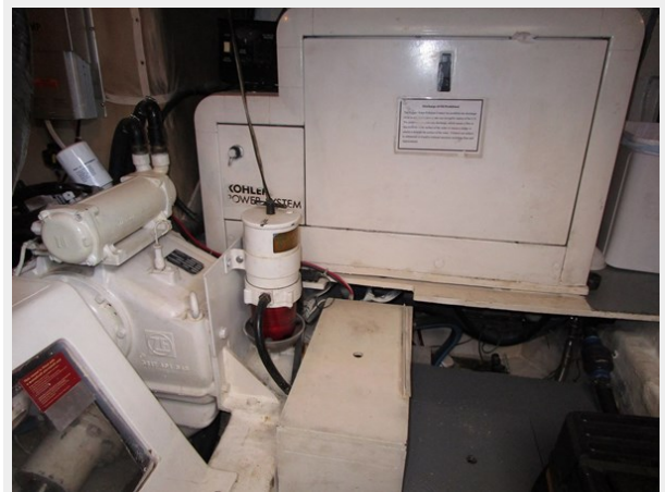
Engine Room Forward
