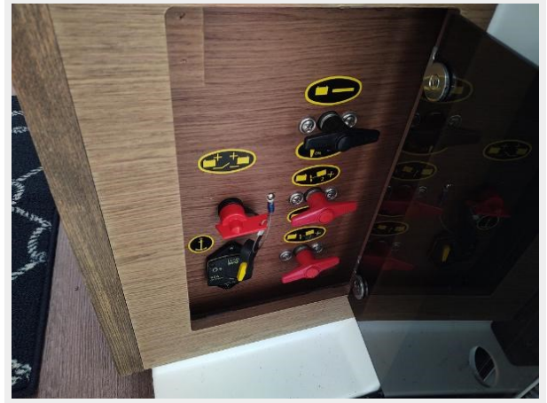
Knot Shore Battery switches
