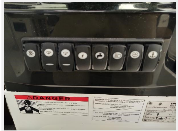
Knot Shore Switch panel
