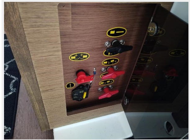
Knot Shore Battery switches
