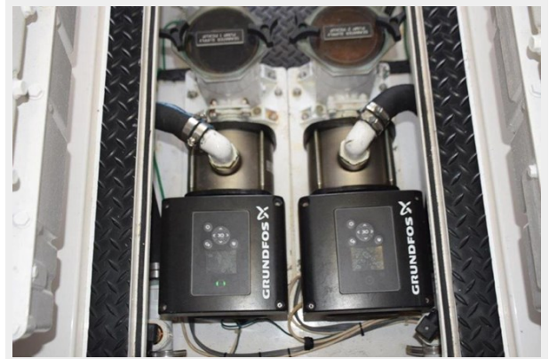
Central Seawater System
