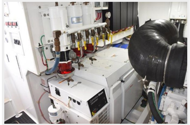
Generator and Primary Fuel Filters
