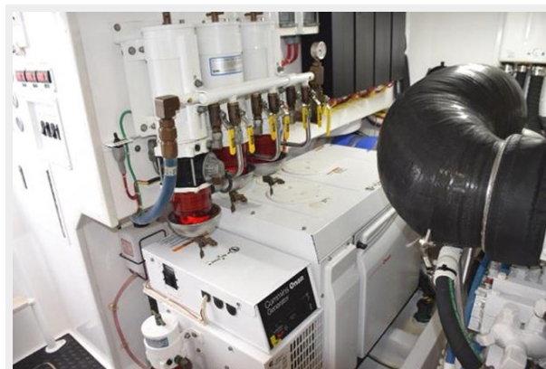
Generator and Primary Fuel Filters
