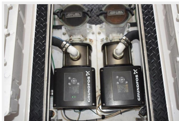
Central Seawater System
