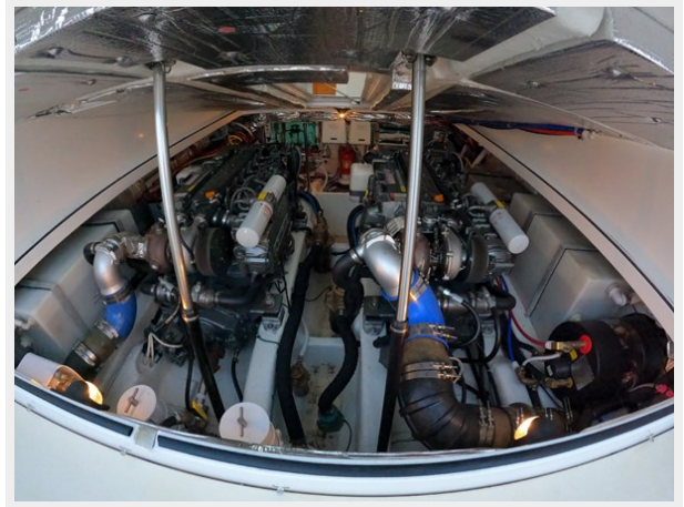
Engine Room w Twin 440's
