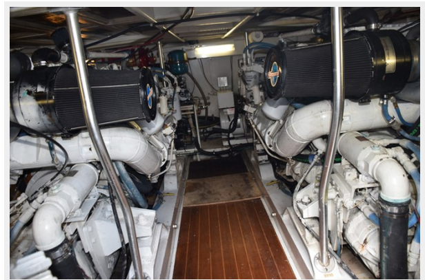
Engine room, Detroit Diesel 8v92s
