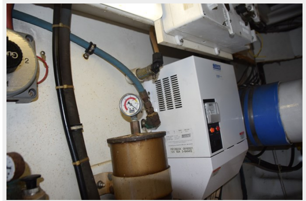
Aft engine room
