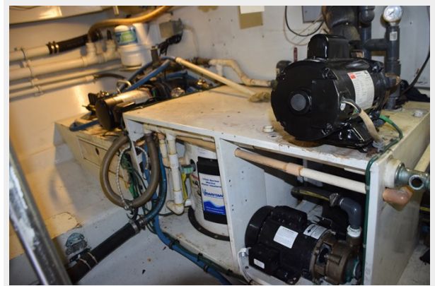
Forward engine room
