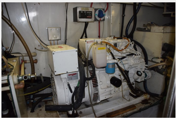
Newer Northern Lights generator
