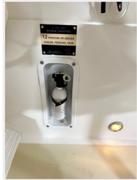
Fire Extinguisher Recessed Mount at Helm
