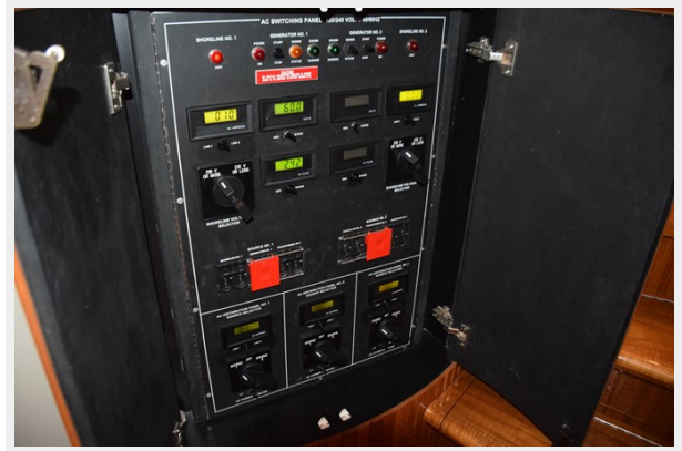
Master Electrical Panel on Companionway
