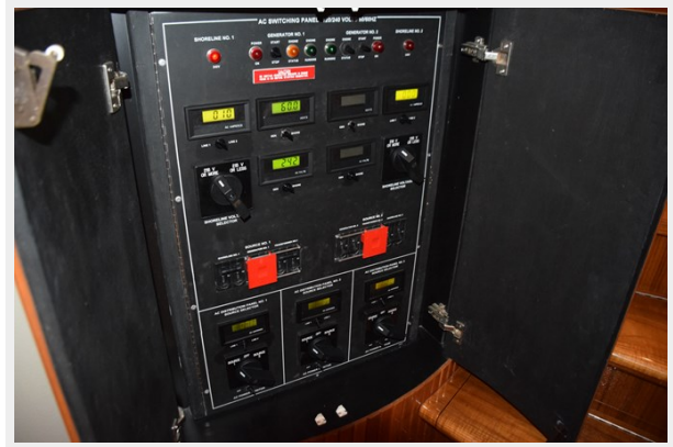
Master Electrical Panel on Companionway
