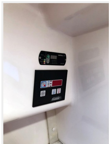
AC and Inverter Controls
