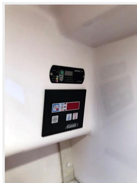
AC and Inverter Controls
