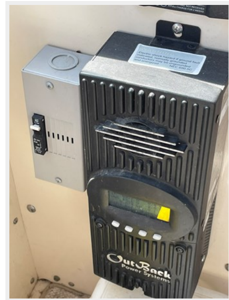
Solar panel controller
