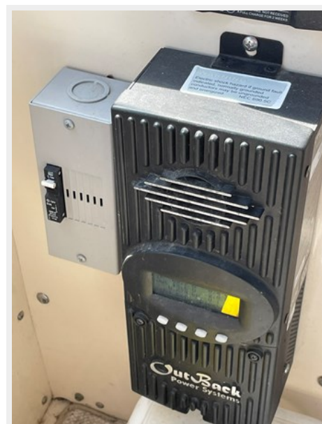
Solar panel controller
