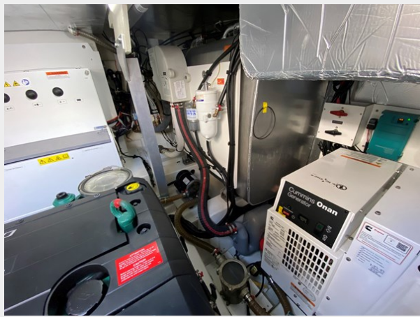
Engine room fwd
