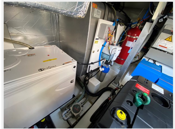
Engine room stbd fwd
