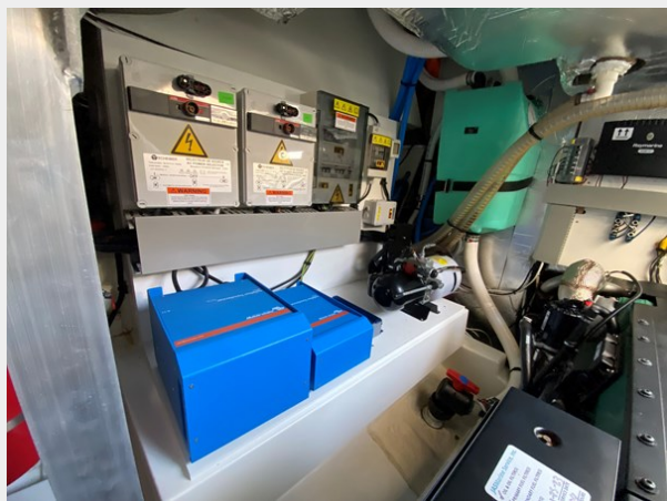
Engine room stbd
