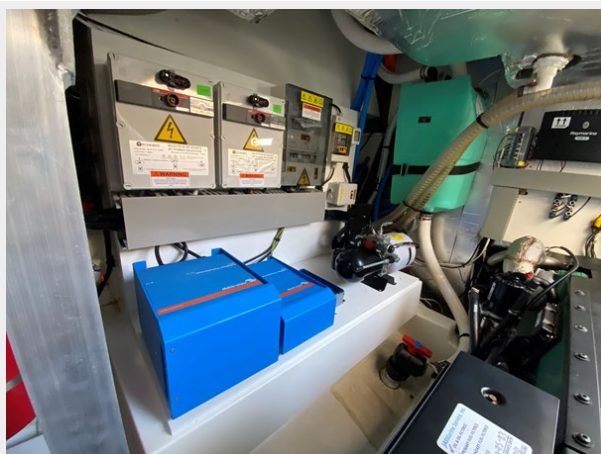
Engine room stbd
