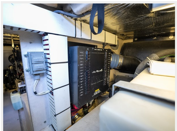
Main DC breaker panel
