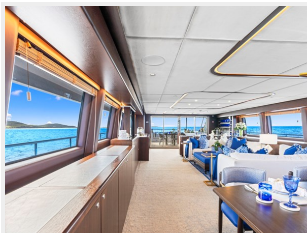
Main Salon Starboard TV Installation
