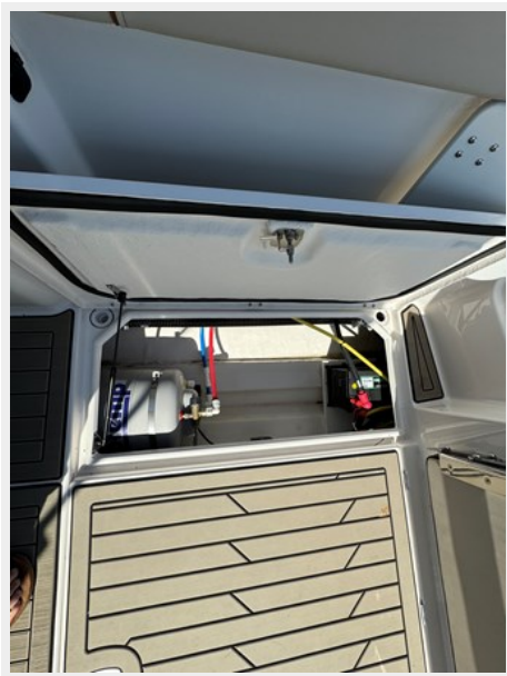
Hot Water Tank
