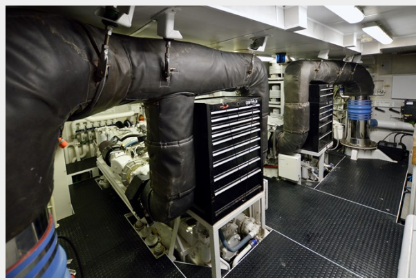
2001 DESTINY 98 ENGINE ROOM 2
