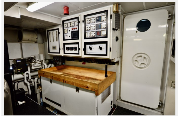
2001 DESTINY 98 MECHANICAL ROOM
