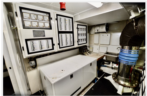
2001 DESTINY 98 GENERATOR - ELECTRICAL PANEL
