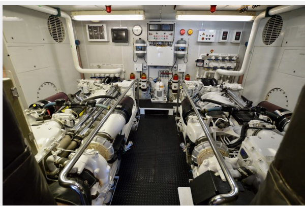
2001 DESTINY 98 ENGINE ROOM
