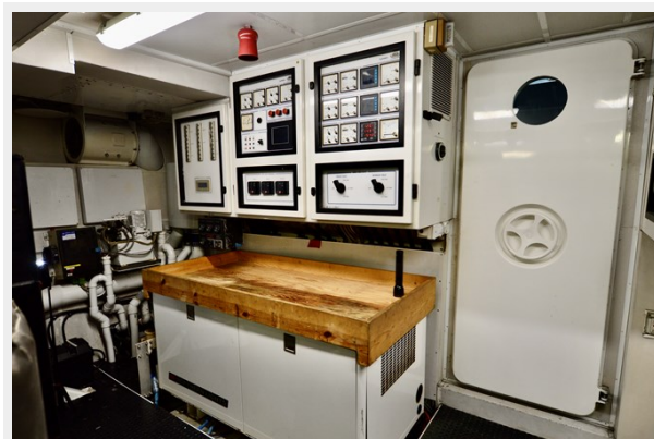
2001 DESTINY 98 MECHANICAL ROOM
