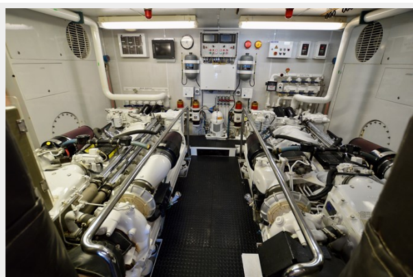
2001 DESTINY 98 ENGINE ROOM
