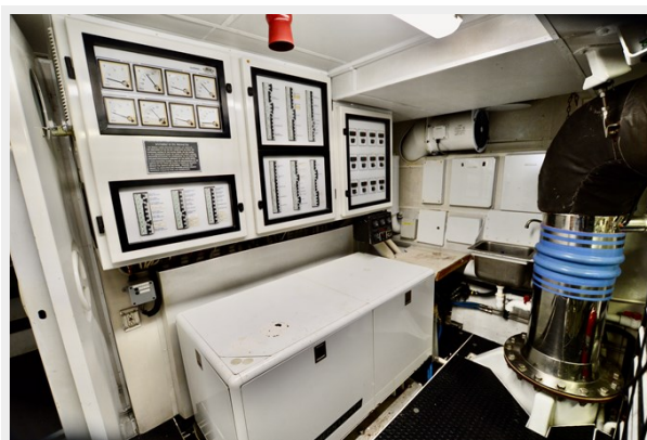
2001 DESTINY 98 GENERATOR - ELECTRICAL PANEL
