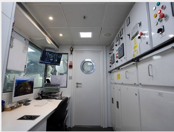
DFLY ENGINE ROOM-3346
