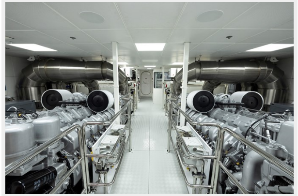
DFLY ENGINE ROOM-3308
