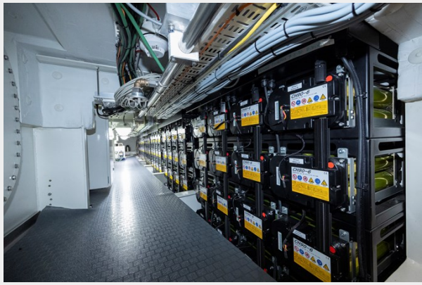
DFLY ENGINE ROOM-3290
