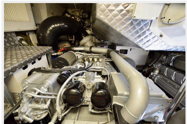
2017 PERSHING 70 ENGINE ROOM 4
