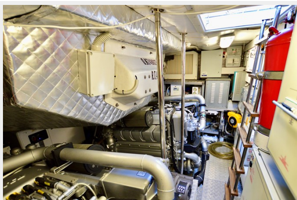
2017 PERSHING 70 ENGINE ROOM
